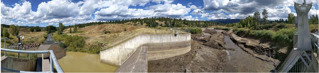
Figure 34. Evidence of sediment removal activities on the upstream side (image-right) of the Oso Diversion Dam on the Navajo River.
